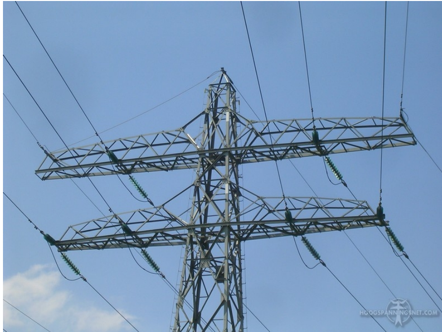
Image 1: Dutch high voltage mast carrying one line on each side 1 .
