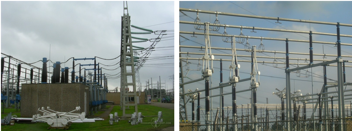
(a) Line termination at circuit breakers.
